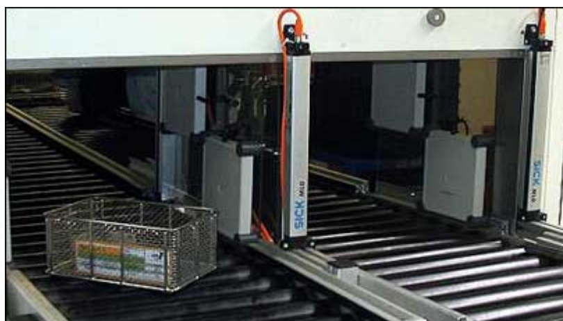
At each juncture in the process, RFID interrogators read a carrier's tag, helping to make sure the appropriate program is being used to wash the parts inside the bin.
